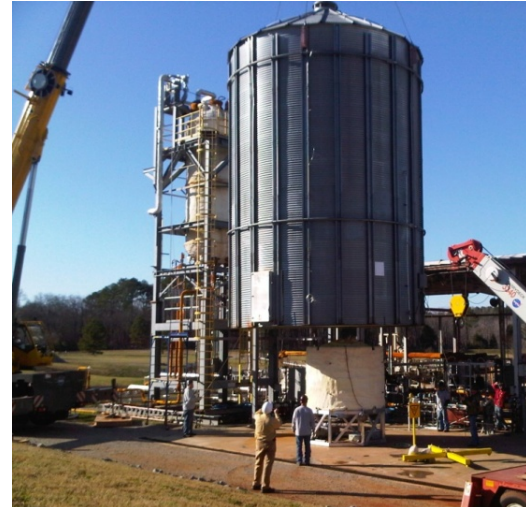
2.4-meter tank with insulation at MSFC Test Stand
